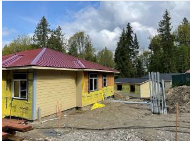
Community building and site electrical conduit
