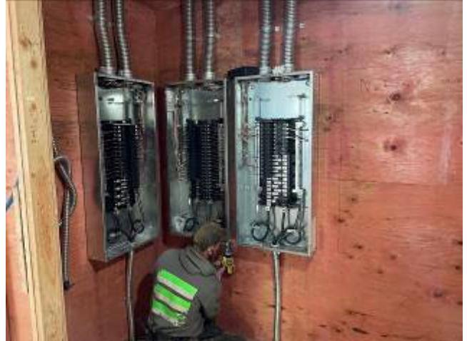
Community building electrical panels
