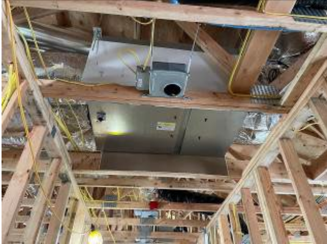
Community building HVAC
